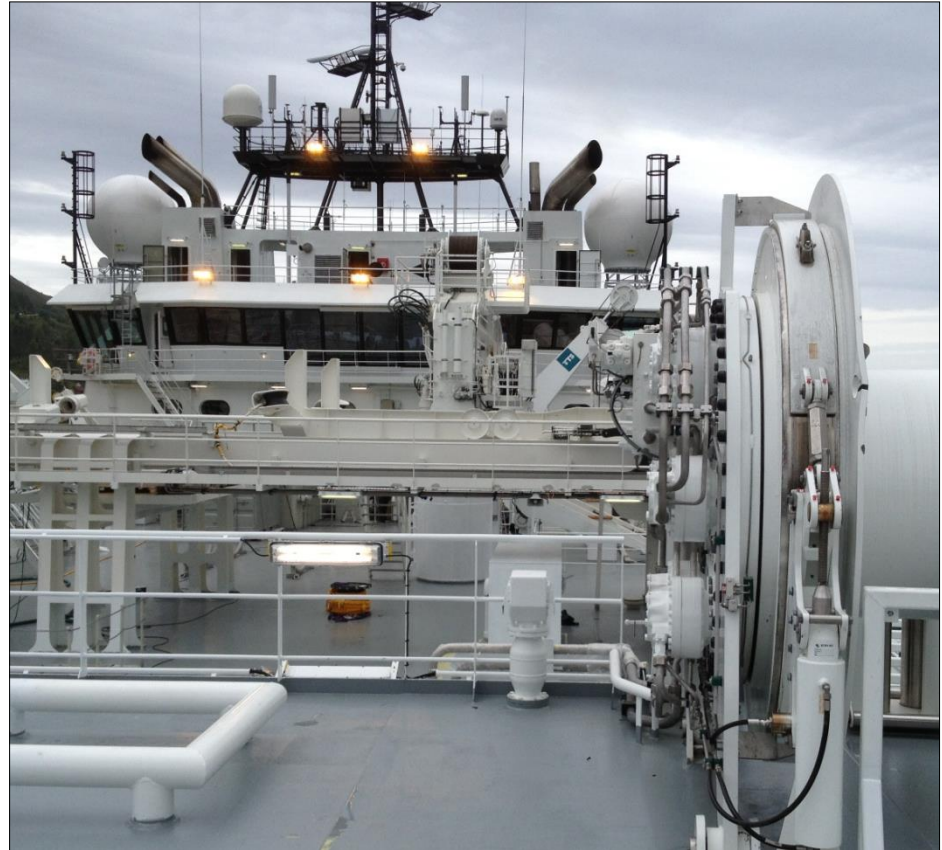
Sanco Swift Seismic Vessel PYPLOK® installed by Kleven Yard in Norway
